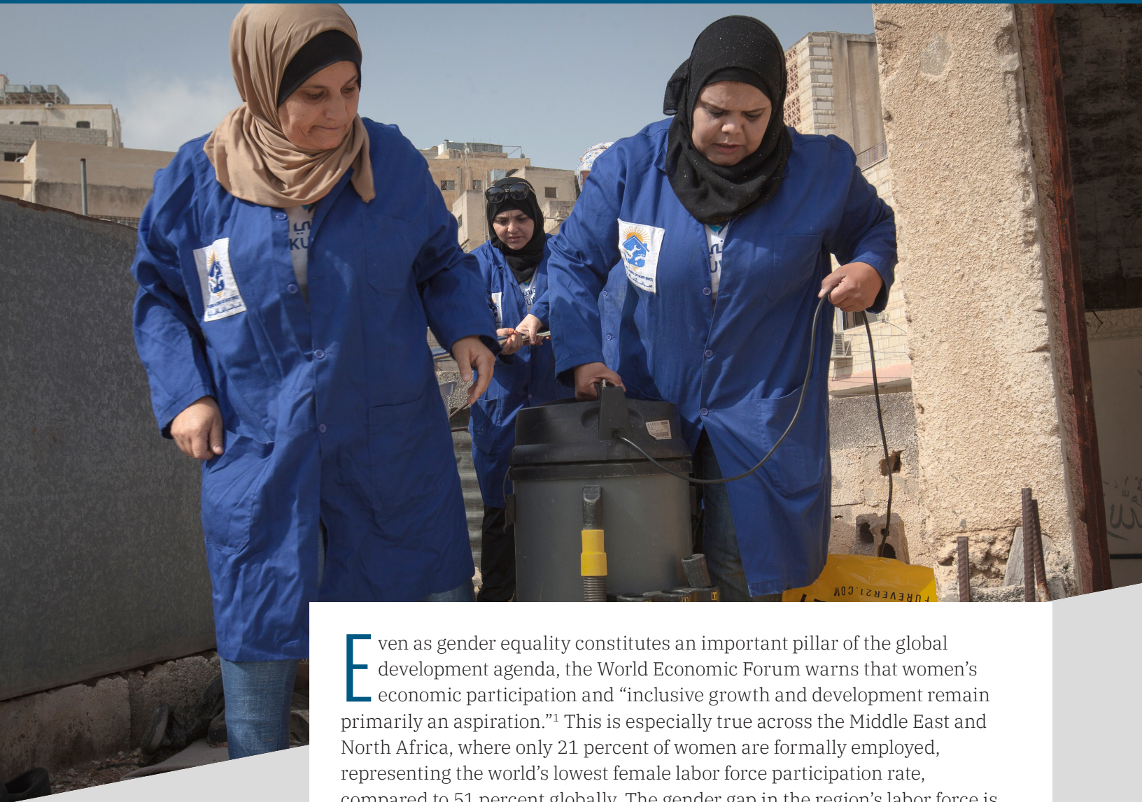
Jordanian women plumbers work on a religious school rooftop as part of a U.S.-sponsored program. Photo: Sebastian Castelier/Shutterstock.com
